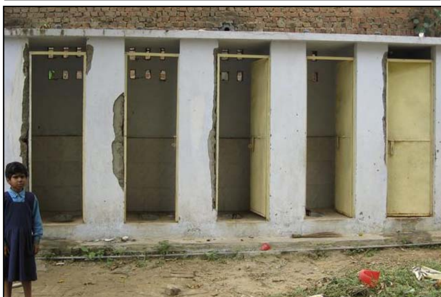
A typical bathroom at a school that Water Centric works with.
